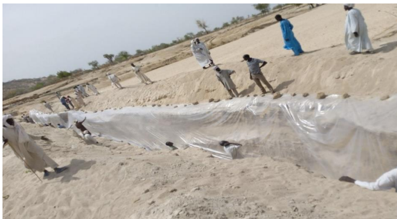
Fig 2: Plastic Sheet To Block Water Losses
