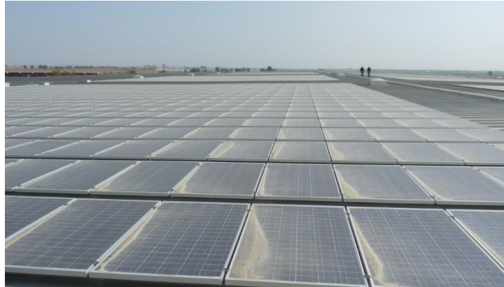
Figure 1: Dust Accumulation on The Surface of Solar Panels
